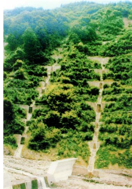
(b) Series of debris-resisting barriers along the drainage line (Photo from Lo 2000)
