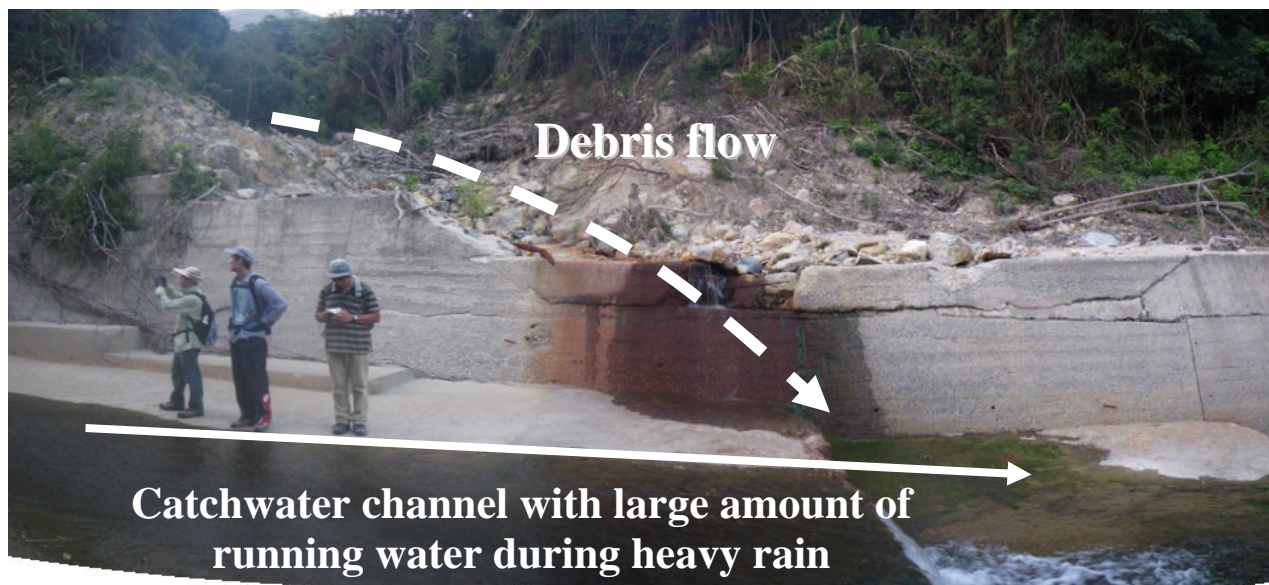
Figure 37: Debris flow entering catchwater channel (Note: The June 2008 Shek Pik No. 1 debris flow is shown; the debris flow turned into a debris flood after entering the catchwater channel)
